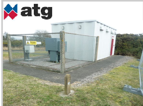
Sub Station at LLWR
